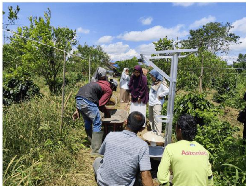
Gambar 2. Instalasi perangkat Automatic Weather Station berbasis IoT di kebun kopi mitra
